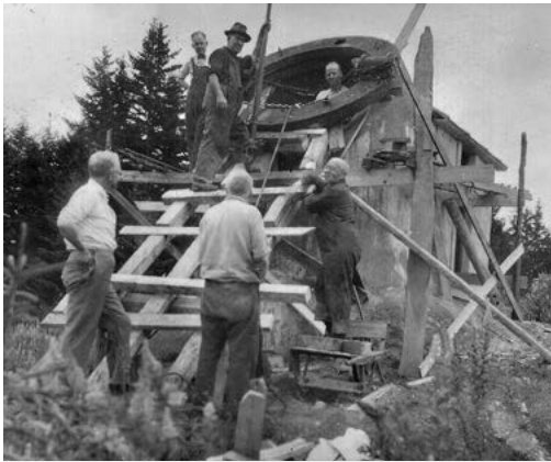
Jacking the heavy RA ring into position during the Porter Turret's construction. The telescope could only have been built in a place like Springfield, where the Jones & Lamson Machine Company, employer of Porter and others, afforded members the means to machine large parts.
